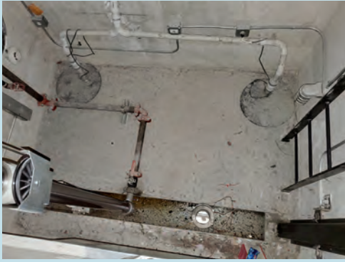
Construction dust from an elevator's installation 15 years prior
